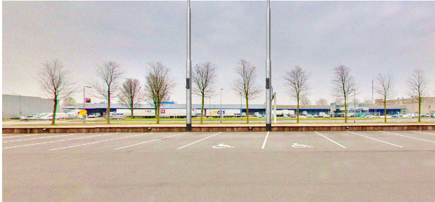
Charging lamppost with internal payment terminal 2 x EV lamp post with payment terminal (type E- LOADER LAMP 22 Kwh TERM)
