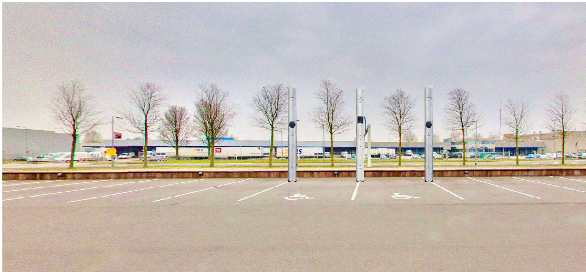
The charging lamppost with central payment terminal EV central payment terminal + 2 x E-loader 22 Kwh Expandable up to 20 charging stations
